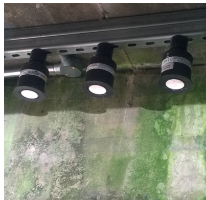
3 dBi HART transducers Monitoring Sluice Levels
